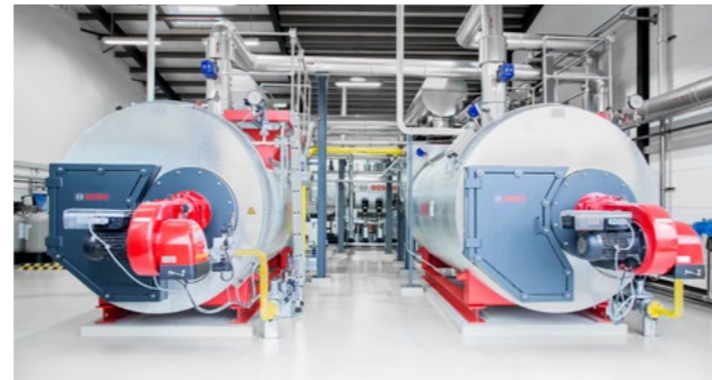
The two efficient Bosch steam boilers supply a total of up to 8 t/h of steam.
