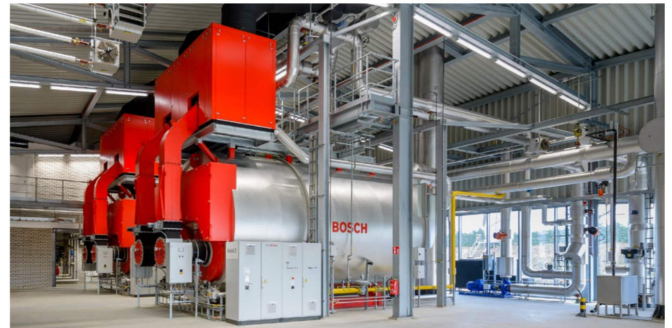
The NO x values are under 50 mg/Nm 3 at the customised boiler system in the Pieter Wiersma heating plant.
