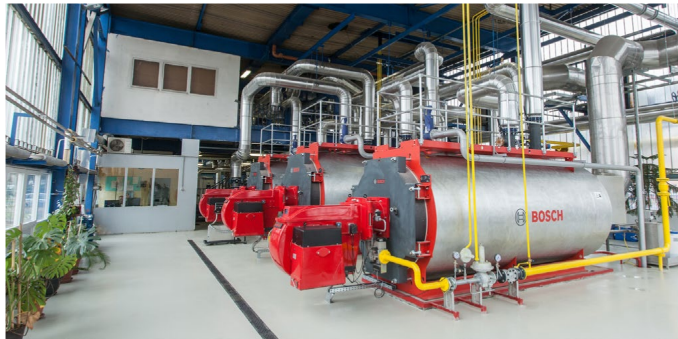
Brought up to current state-of-the-art technology with new Bosch heating boilers.
