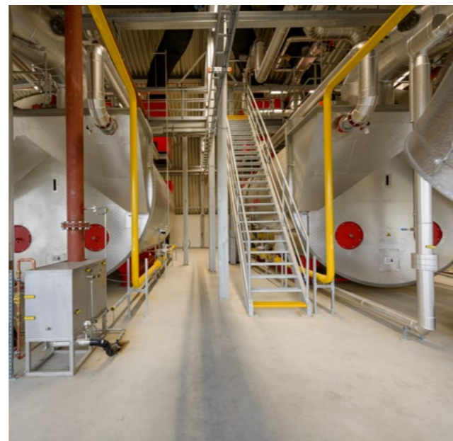
Flue gas heat exchanger ECO
